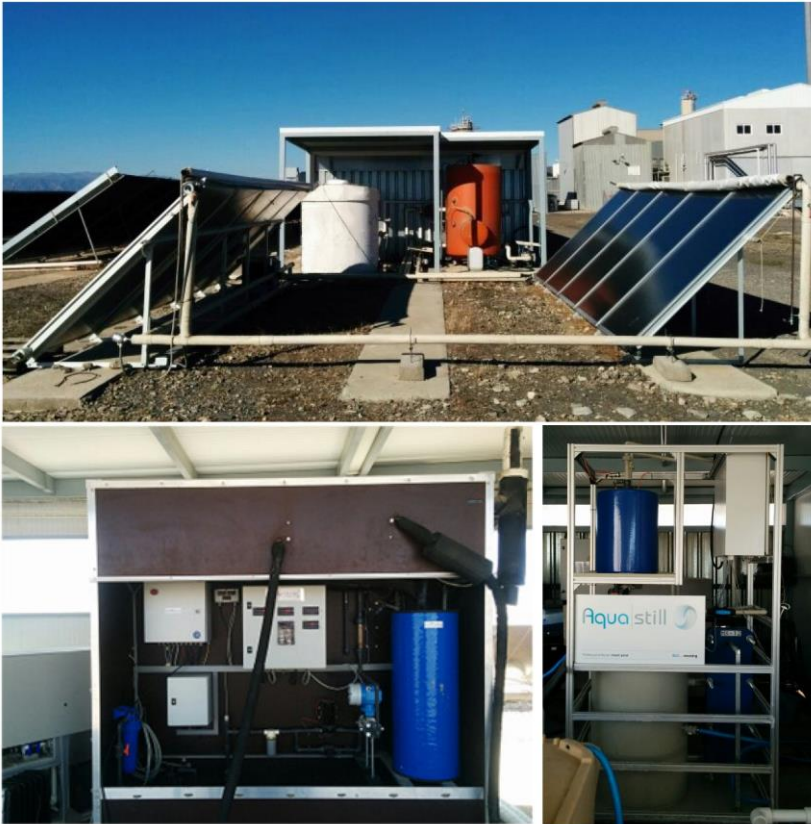
SMD pilot plant at PSA. From top to bottom and from left to right: solar field, Solar Spring module and Aquastill module.
